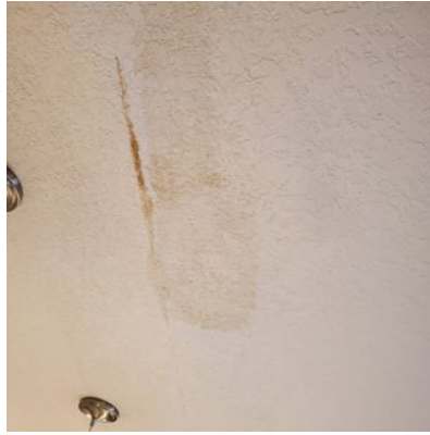
Stain on the kitchen ceiling
