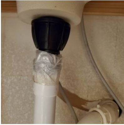
Improper repair of a drain pipe under the guest bathroom lavatory
