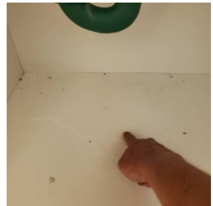
Leaking pipe under the master bathroom lavatory
