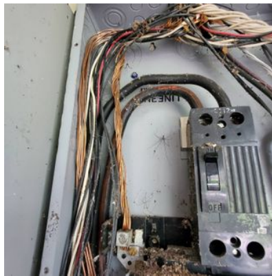
Improper grounding inside the main panel
