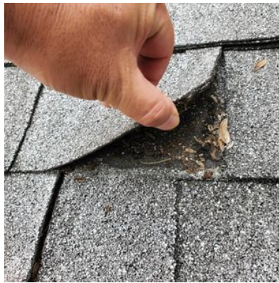
Loose shingles at multiple locations
