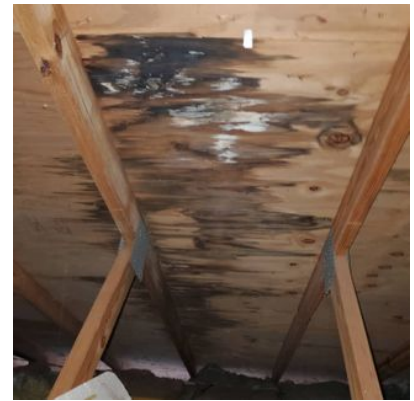
Stain on the underside of roof decking above the garage
