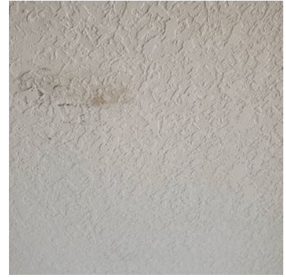
Stain on the garage ceiling
