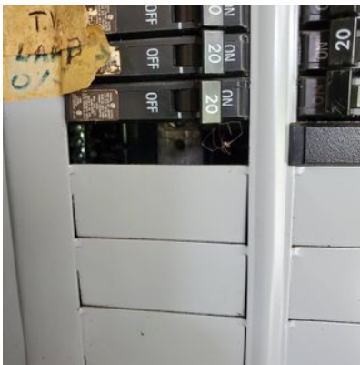
Open socket at the main panel
