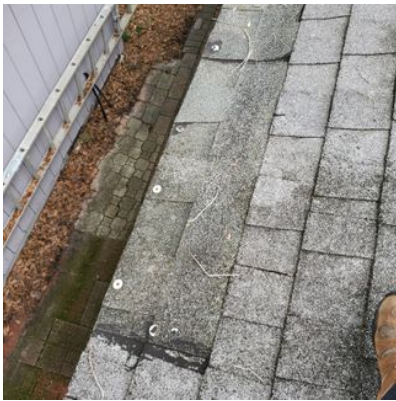
Exposed fasteners on the right side of the roof
