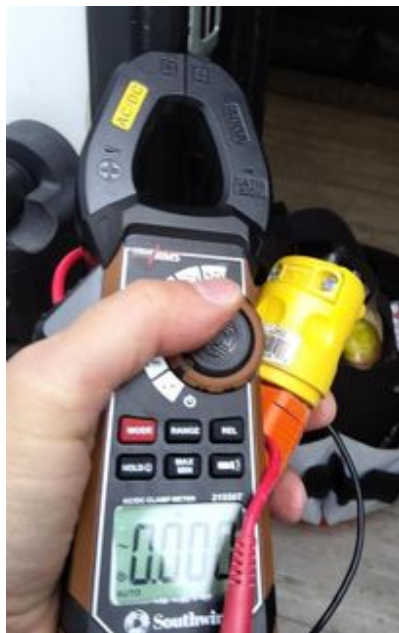
No Excessive Voltage at Entrance Door
