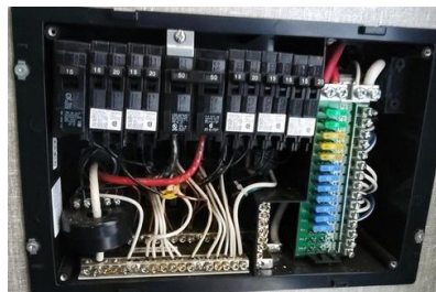
Electrical Panel - Cover Off
