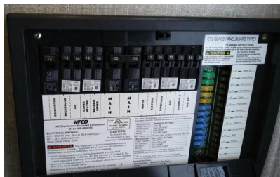
Electrical Panel - Cover On
