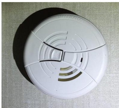
Garage Smoke Detector - Front
