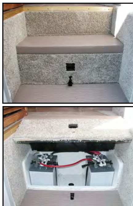
Figure 7-3. Stairwell (Top) and Battery Storage Underneath (Bottom)
