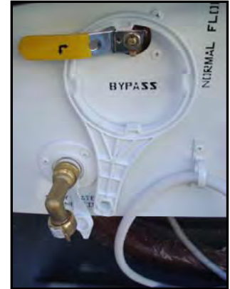
Figure 11-8. Water Heater Bypass System
