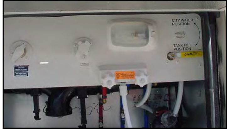
Figure 11-6. City Water Connection
