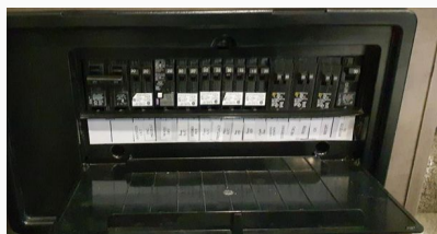
Electrical Panel - Cover On
