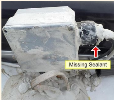
Curbside Roof Junction Box
