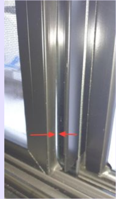
Emergency Exit Window Screen
