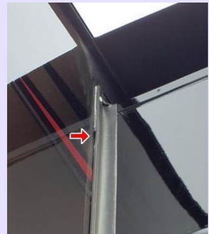
Upper Rear of Rear Curbside Slideout Seal
