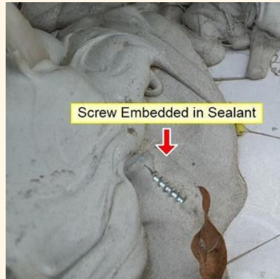
Screw near Junction Box
