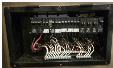
Electrical Panel - Cover On
