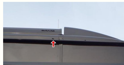
Uneven Sealant Above Curbside Entrance Door
