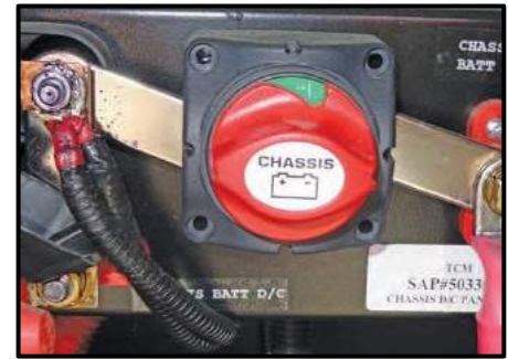
Figure 9-15: Engine Battery Disconnect Switch
