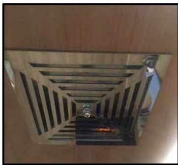
Figure 3-2: Outgoing Air Vent
