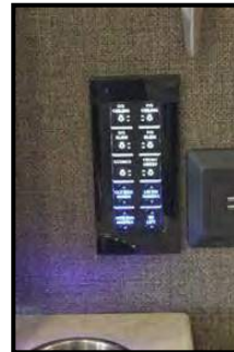
Figure 6-5: Television Lift Control Panel (located in the living room slide-out box)
