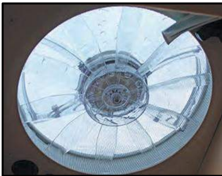
Figure 14-4: Overhead Vent Fan
